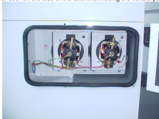
View of motors once lower door is opened.
